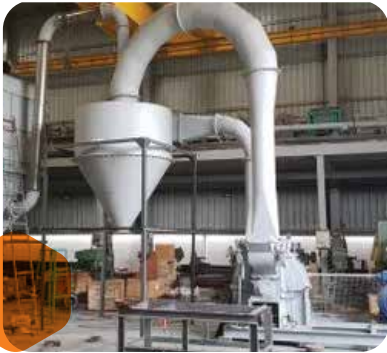
Coal Feeding & Ash Handling System
